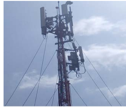
Figure 3.2: Node B at Sokoban Site
