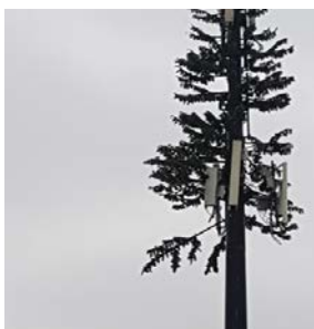
Figure 3.1: Node B at KNUST Brunei Site
